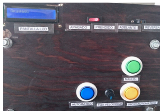
Figura 6.1 Panel de Control.
